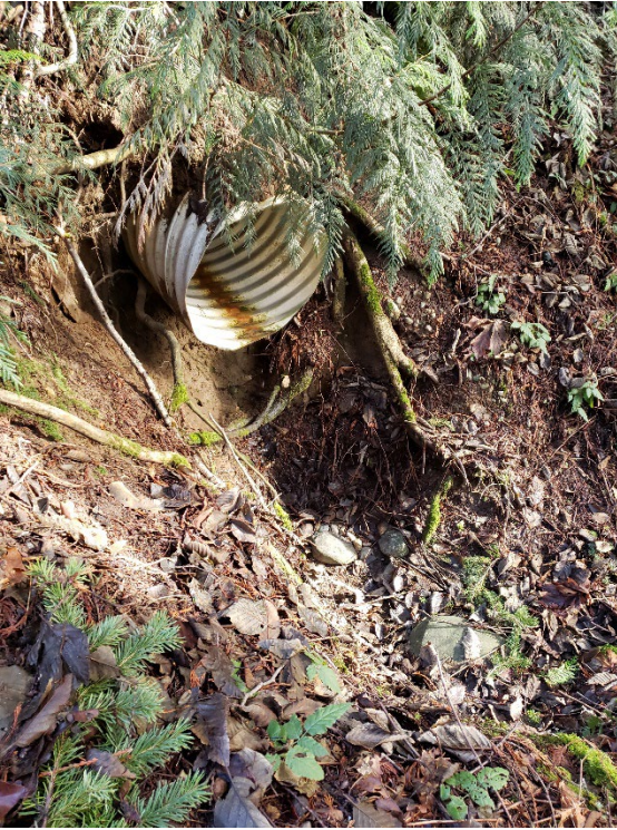
Photograph 5. Outfall of the downstream culvert to culvert 4 with downcutting at station 30+75.
