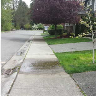
Example of groundwater seepage
