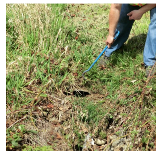
Roadside ditch in need of maintenance. Vegetation is blocking inlet to pipe.
