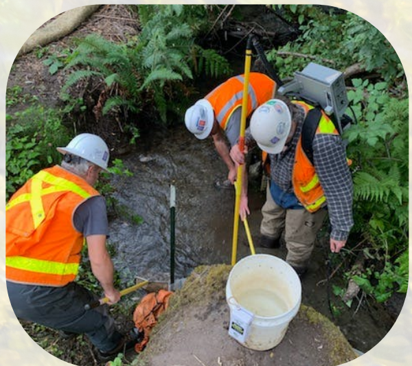
Removing fish from the stream before diverting the creek for installation of the new culvert.
