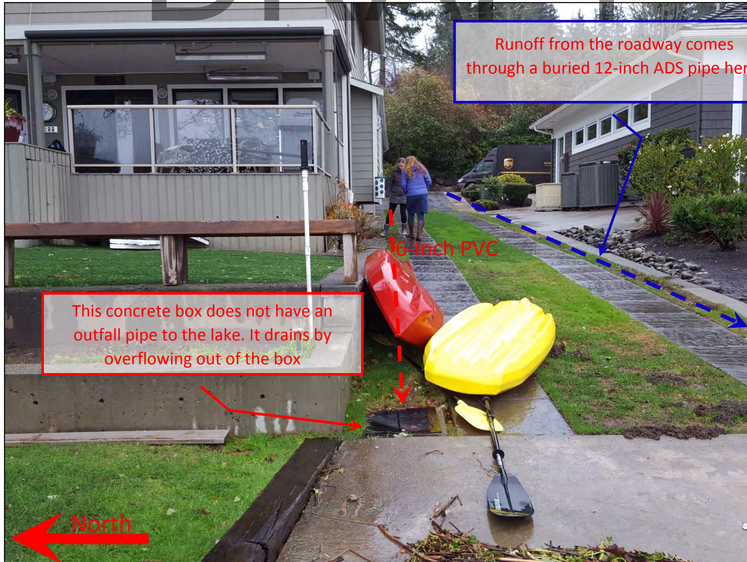
Picture 6 – This picture shows the 6-inch pipe continuing to the catch basin/concrete box at the lake adjacent to the boat launch at house #439. During our visit the box was flowing out of the grate from the top and flowing down the boat launch. The connected 6-inch pipe was under over 8-inches of water. (Looking east towards home #439) *The exact location of the 6-inch PVC line in respect to home #425 and 439 and the structure at the lake is assumed to be in this location.
