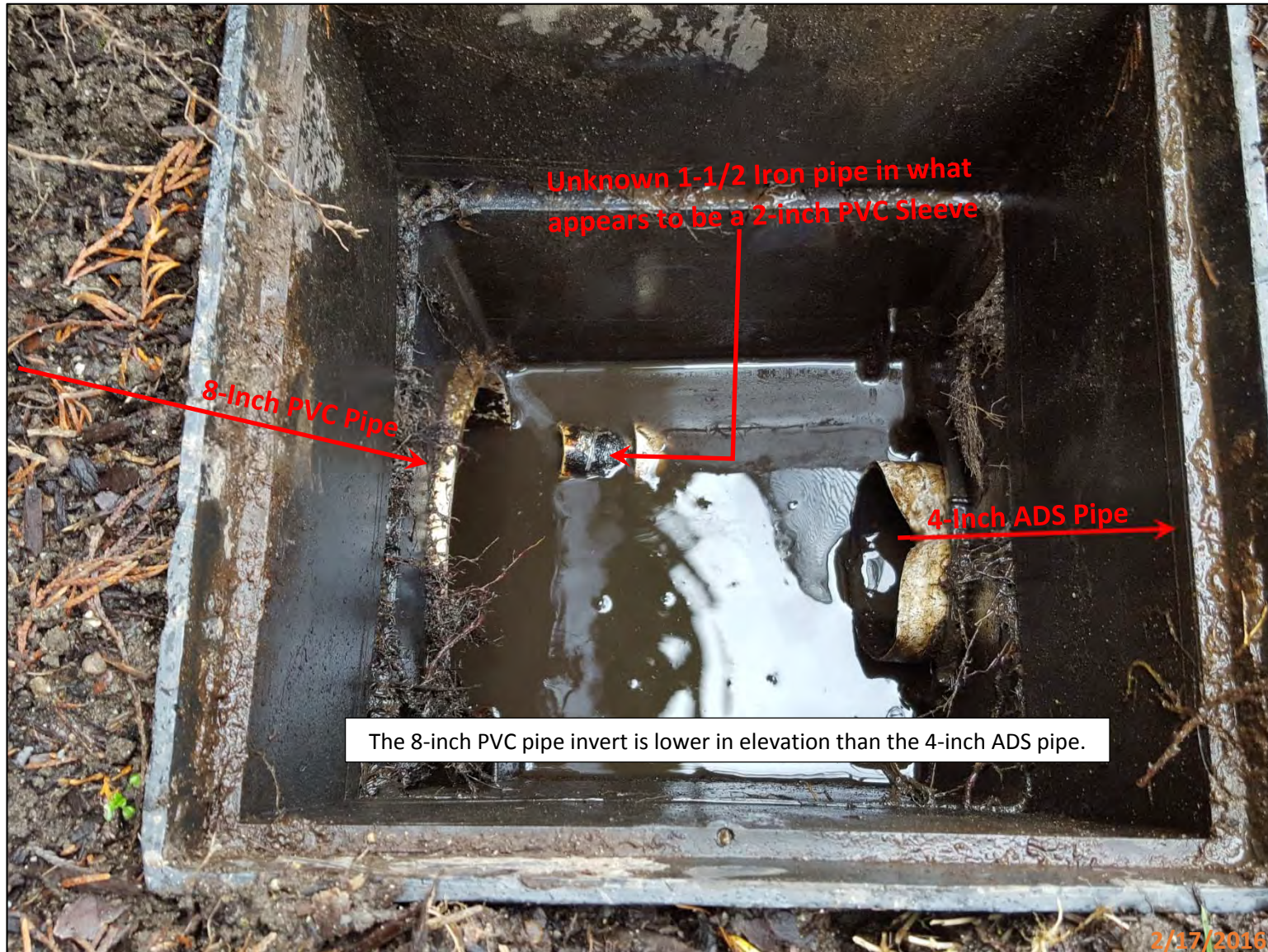
Picture 10 - This picture shows the yard drain after to the vactor truck cleaned it out. The 8-inch PVC pipe shown comes from the ELST trail drainage ditch. The 4-inch ADS pipe appears to be connects to a nearby homeowner drainage system to the east on East Lake Sammamish Shore Ln SE. The 4-inch ADS pipe was not cleared out or viewed with a pipe camera. This yard drain was completely filled with water to the rim of the structure prior to cleaning it out. See picture 9 to view this structure prior to it being cleaned out.
