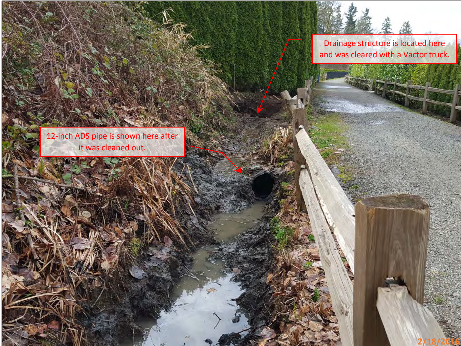
Picture 2 - This picture shows the drainage system from Picture 1 after it was cleared out with a vactor truck. This pipe is lower than the ditch which causes it to backflow. (Looking south on the trail adjacent to 1428 E Lake Samm Shore Ln SE)
