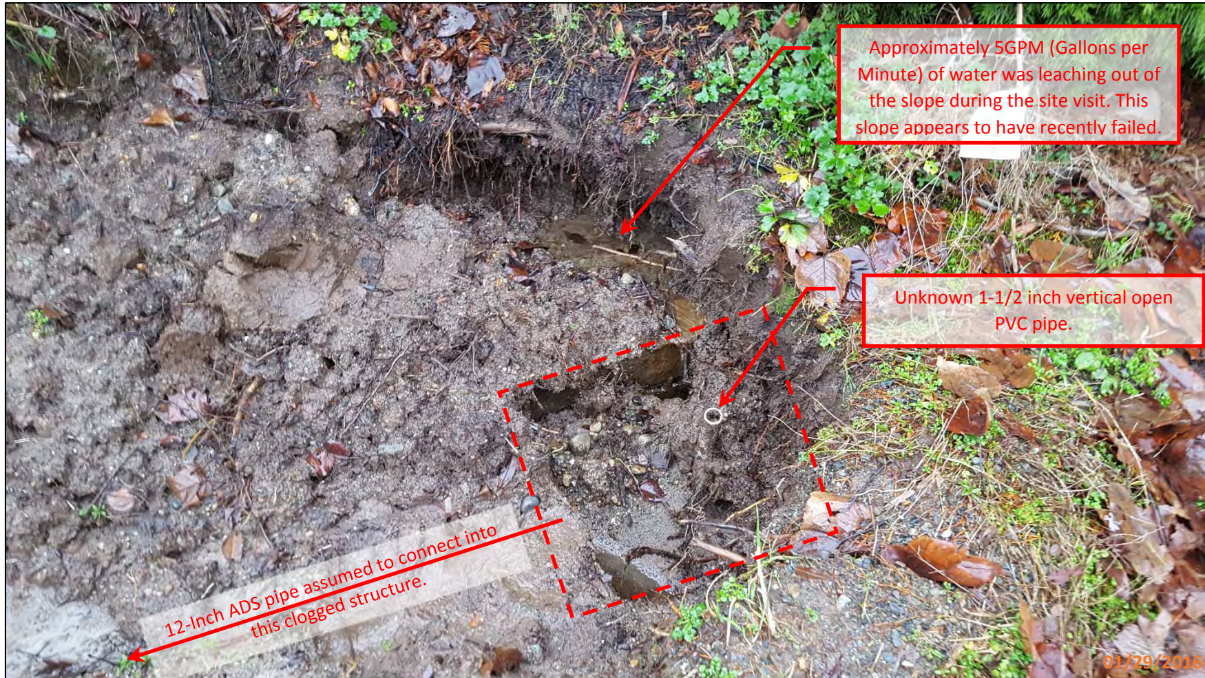
Picture 9 – This picture shows a clogged structure that connects to the 12-inch ADS pipe in the drainage ditch on the ELST trail. The slope adjacent and directly east of this structure has failed and clogged the ditch. There is also a minor amount of water leaching out/bubbling up out of the ground at this location. Note: There is also a 1-1/2 diameter PVC pipe sticking up vertically in the structure. This pipe is unknown.
