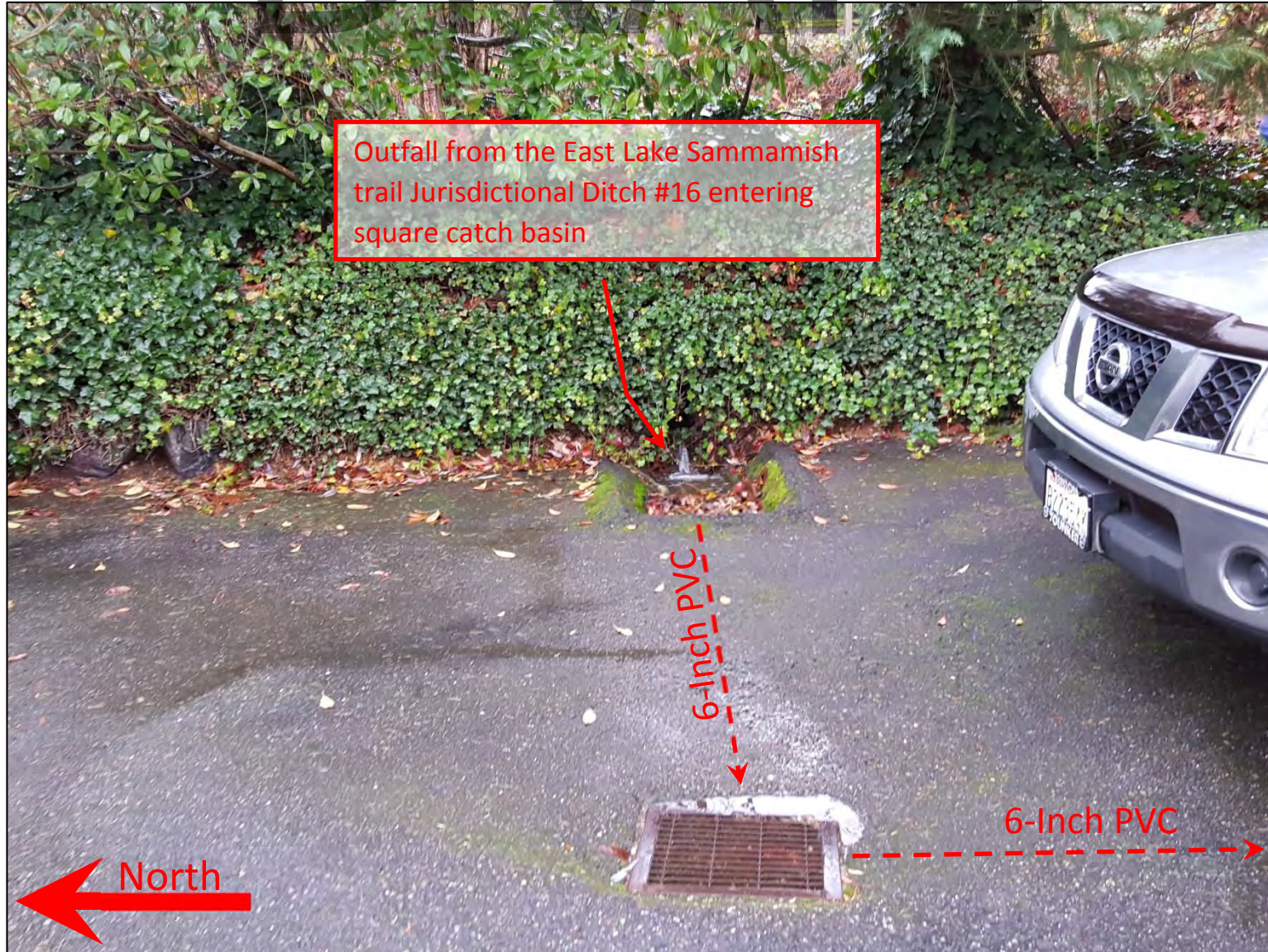
Picture 1 – This picture shows the outfall from the west side of the ELST Trail. This outfall drains Jurisdictional Ditch #16. After entering the catch basin shown the water enters the catch basins shown in this photolog through a 6-inch PVC pipe and ultimately enters Lake Sammamish. (Looking east from East Lake Sammamish Shore Ln NE)
