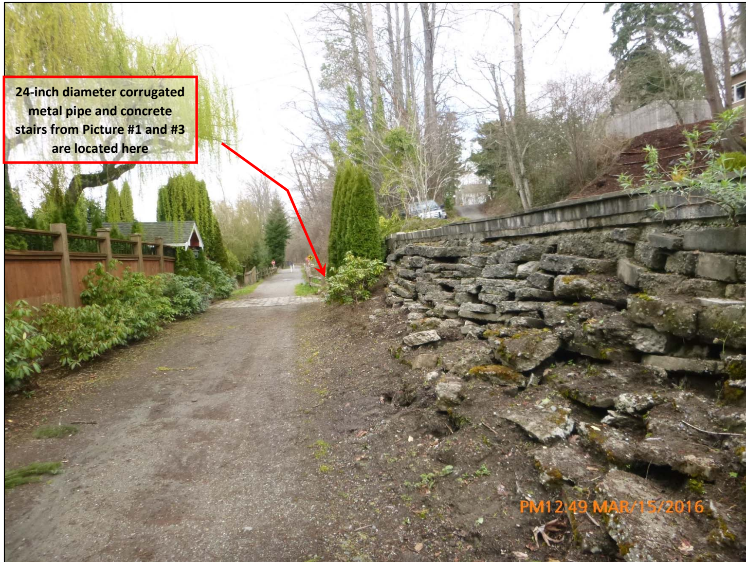
Picture 4 – The pipe continues to the south and appears to potentially travel under the concrete rubble wall. (Looking North)
