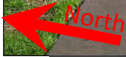
Picture 3 – This picture shows the location that this pipe terminates in the grassy area between the two parcels. The pipe transitions to a perforated PVC pipe at the start of the homeowner’s grass. The pipe ends at the location shown and does not daylight out of the ground. (Looking east between parcels 0777100095 and 0777100105)
