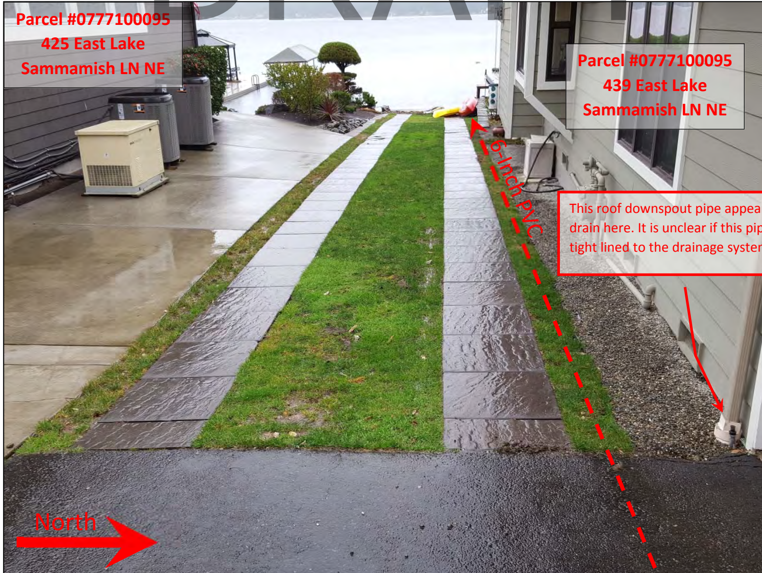
Picture 5 – This picture shows the 6-inch pipe continuing to the lake adjacent to house #439. This picture also shows the downspouts of the house entering a washed rock trench against the home exterior walls. The homeowner indicated water was coming up out of this washed rock trench closer to the lake. (Looking west towards the lake near 439 East Lake Sammamish Ln NE) *The exact location of the 6-inch PVC line in respect to home #425 and 439 and the structure at the lake is assumed to be in this location.
