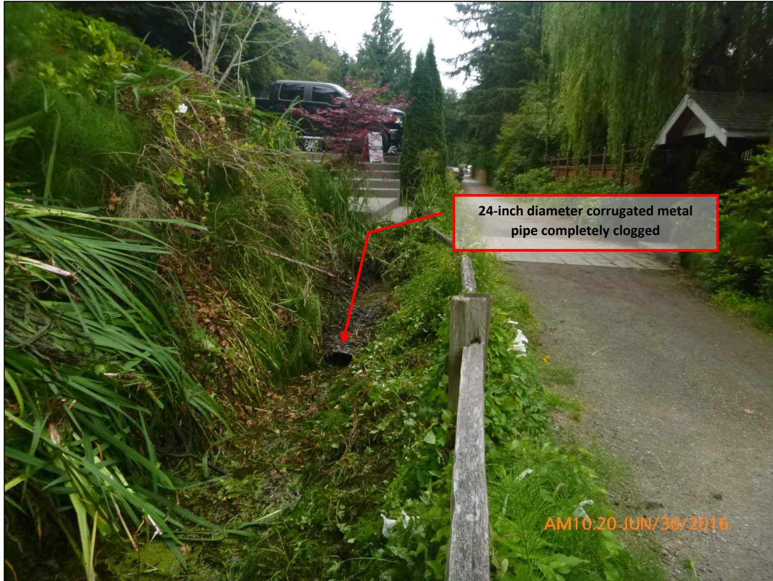
Picture 1 – This photo shows the clogged 24-inch corrugated metal pipe in front of the Hill residence. (Looking south)
