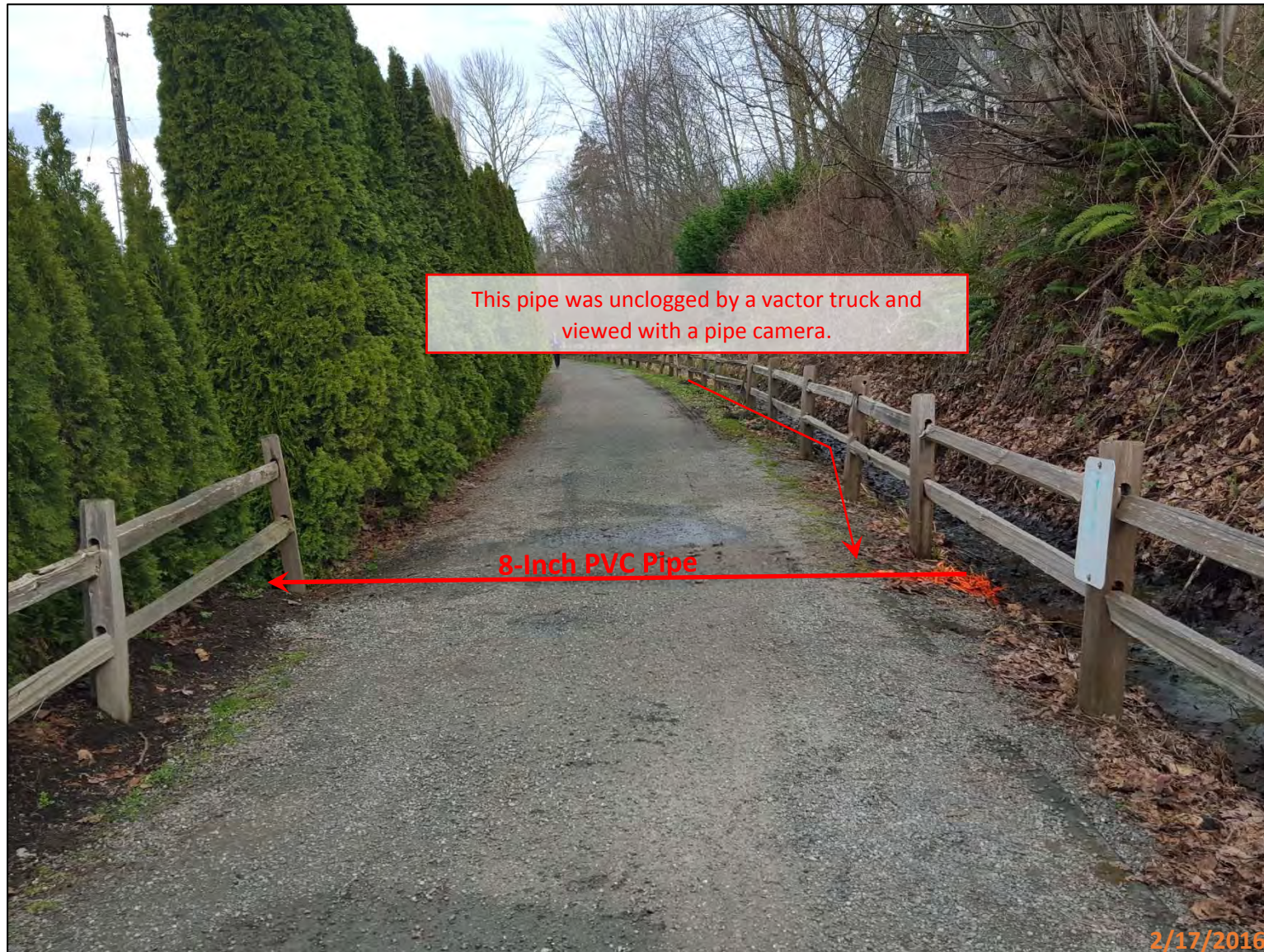
Picture 7 – This 8-inch PVC pipe travels west from the drainage ditch and enters a yard drain in front of 1428 E Lake Sammamish Ln SE. (Looking north)
