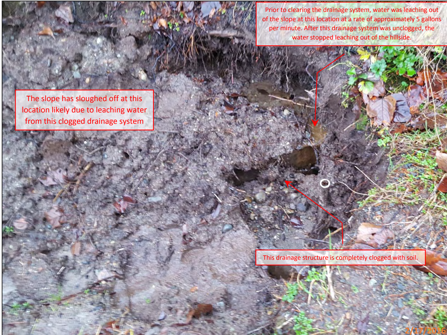
Picture 3 – This picture shows the clogged drainage structure in the trail drainage ditch adjacent to 1428 E lake Sammamish Shore Ln Se. (Looking downward and to the east)
