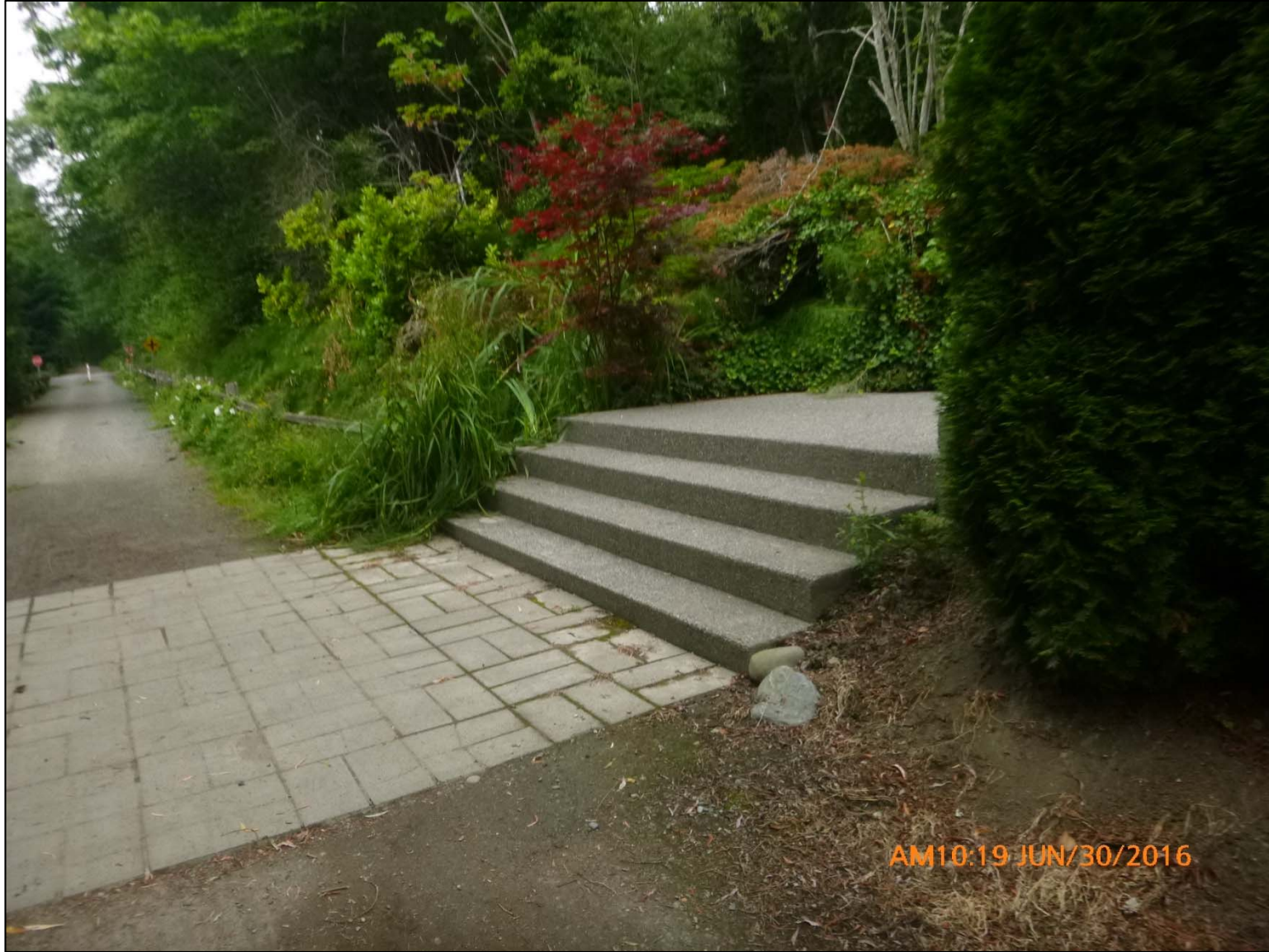
Picture 3 – Concrete stairs directly south of the clogged corrugated metal pipe. The pipe appears to travel southward under these stairs and towards the concrete rubble wall (Looking North)
