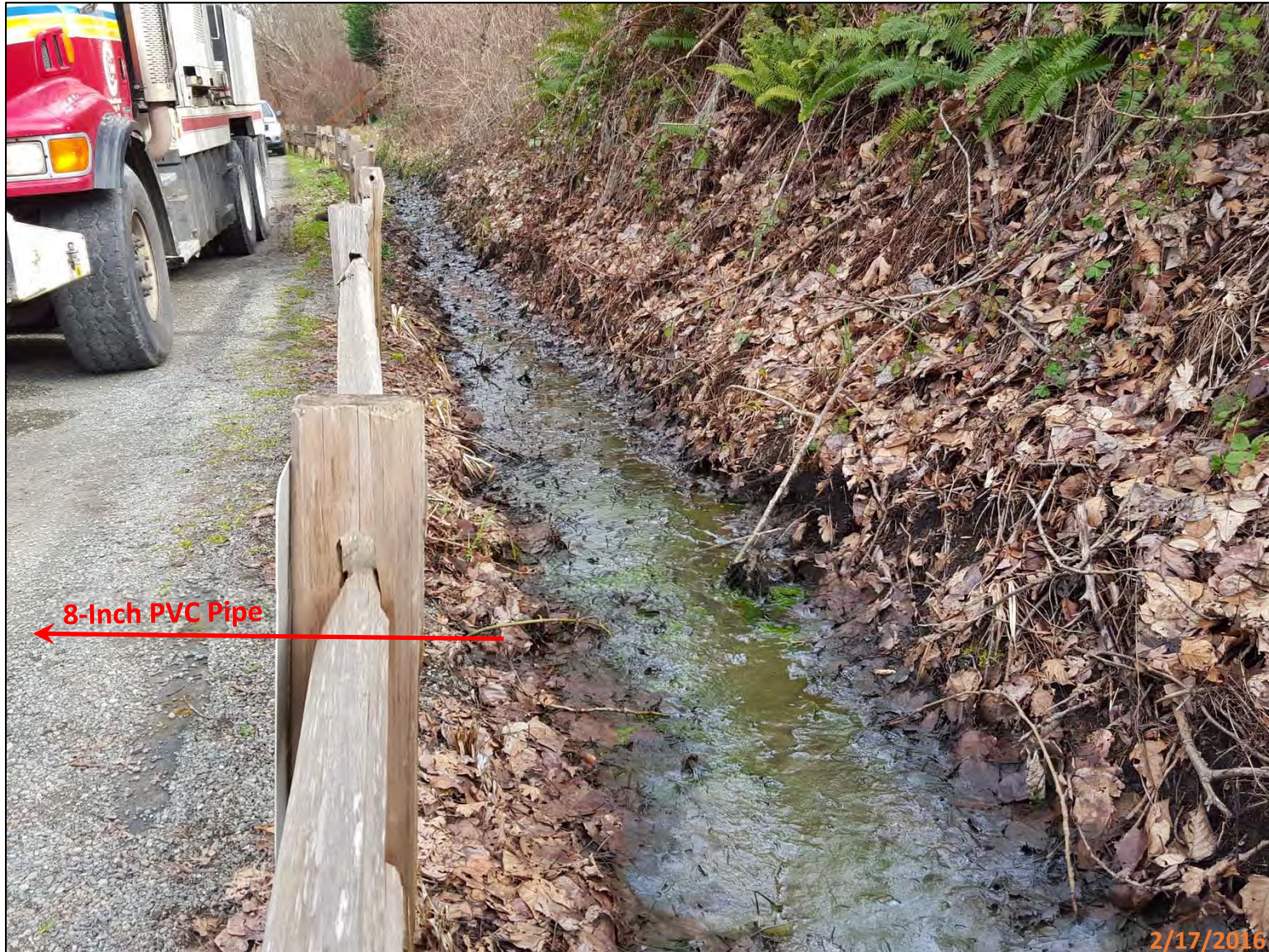
Picture 6 – This picture shows the drainage ditch/wetland approximately 20-to-30 feet north of the drainage system shown in pictures 1-5. This ditch water backflows into the drainage system because the ADS pipe shown in Picture 1 and 2 is lower in elevation than the drainage ditch. There is also an 8-inch PVC pipe that travels beneath the trail and connects to a yard drain in front of 1428 E Lake Samm Shore Ln SE (shown in red). See Picture 7-10 for more information on this drainage pipe. (Looking north)
