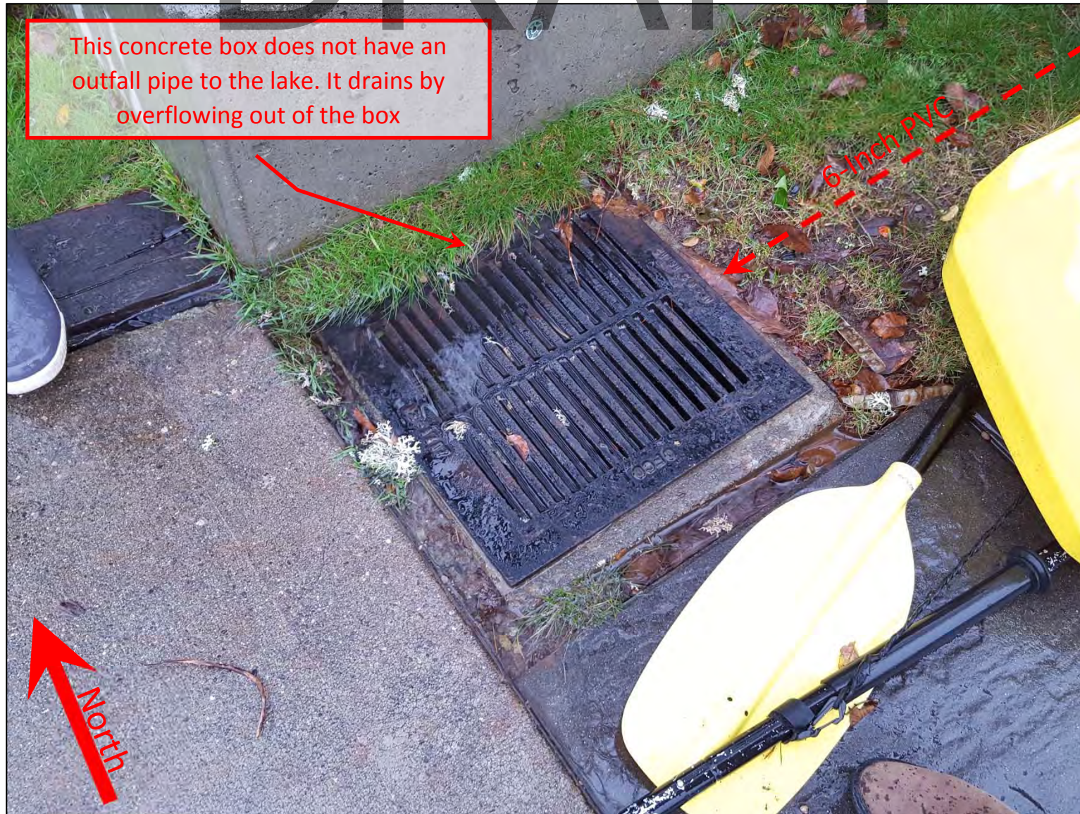
Picture 7 – This picture shows the catch basin/concrete box at the lake adjacent to the boat launch at house #439. During our visit the box was flowing out of the grate from the top and flowing down the boat launch. The connected 6-inch pipe was under over 8-inches of water.
