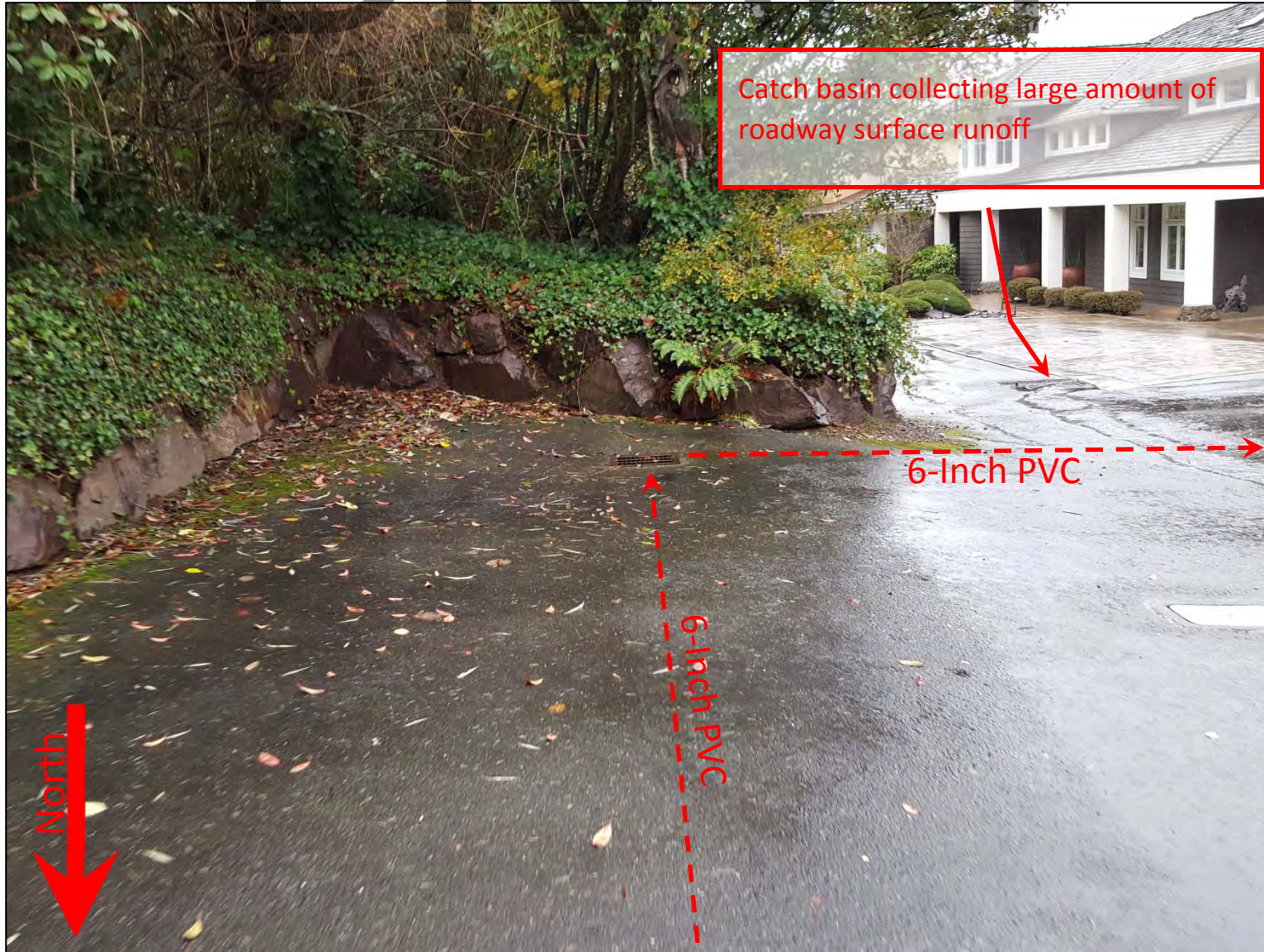
Picture 3 – This picture shows another catch basin on East Lake Sammamish Shore Ln NE. (Looking south from East Lake Sammamish Shore Ln NE)
