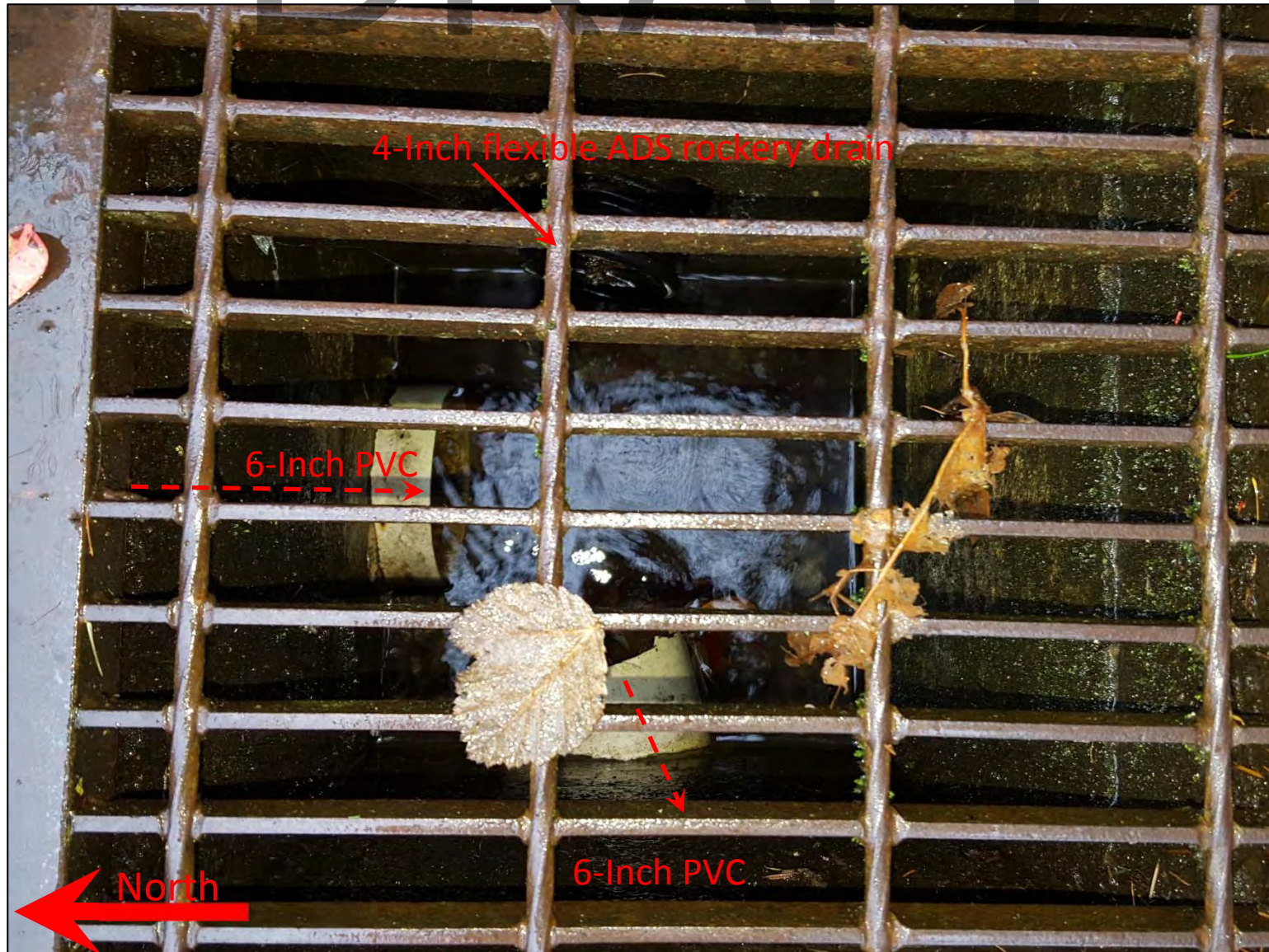
Picture 4 – Looking downward at the catch basin from Picture 3 on East Lake Sammamish Shore Ln NE. The water continues through the 6-inch PVC pipe. The black pipe on the top of the picture is a 4-inch ADS pipe that appears to come from the rockery to the east. (Looking downward and facing east from East Lake Sammamish Shore Ln)
