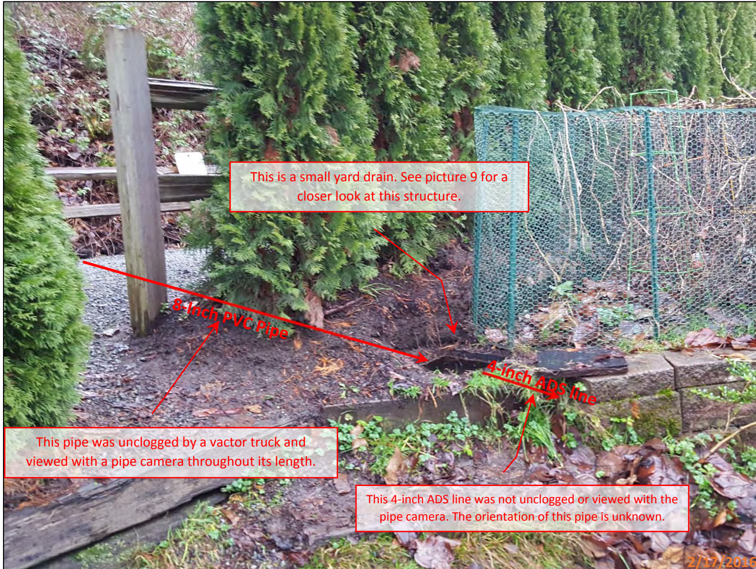
Picture 8 - This 8-inch PVC pipe travels west from the trail drainage ditch and enters a yard drain in front of 1428 E Lake Samm Shore Ln SE. This yard drain was filled to the rim with water prior to the vactor truck cleaning the structure out. This is the location that appears to overflow onto the adjacent private roadway in heavy rain events. This area received a complaint from the Tsilas Residence on 1/19/2016.
