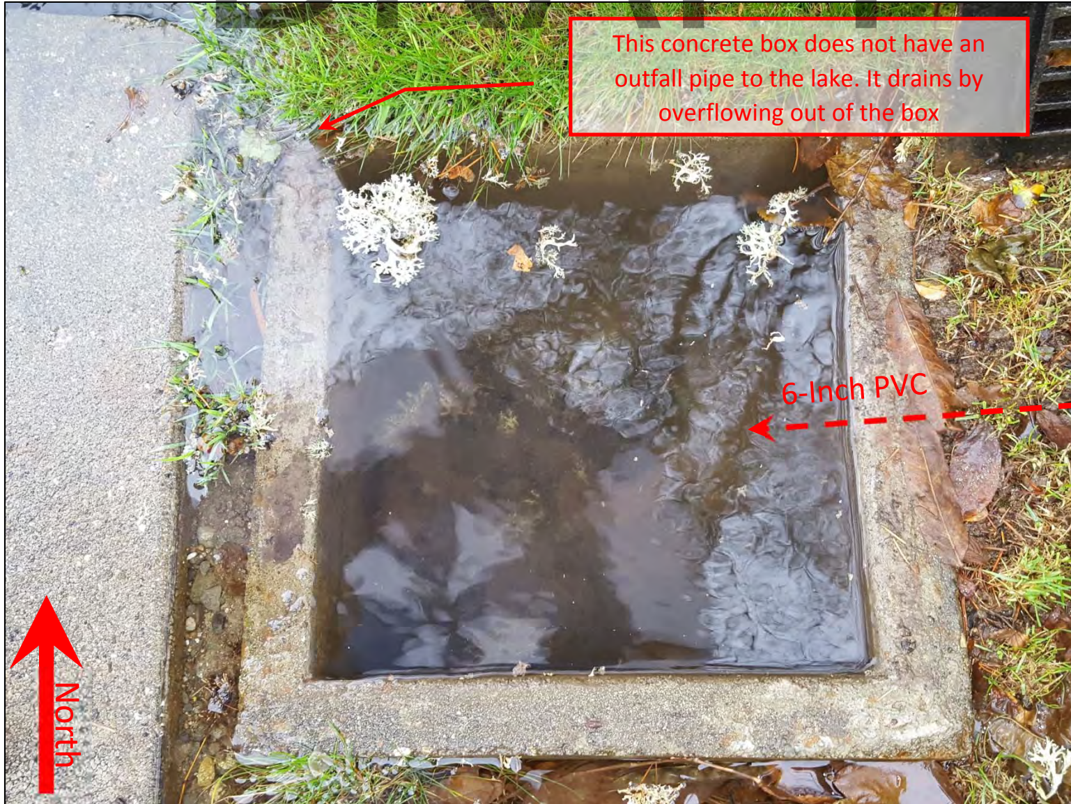
Picture 8 – This picture shows the catch basin/concrete box at the lake adjacent to the boat launch at house #439. During our visit the box was flowing out of the grate from the top and flowing down the boat launch. The connected 6-inch pipe was under over 8-inches of water.
